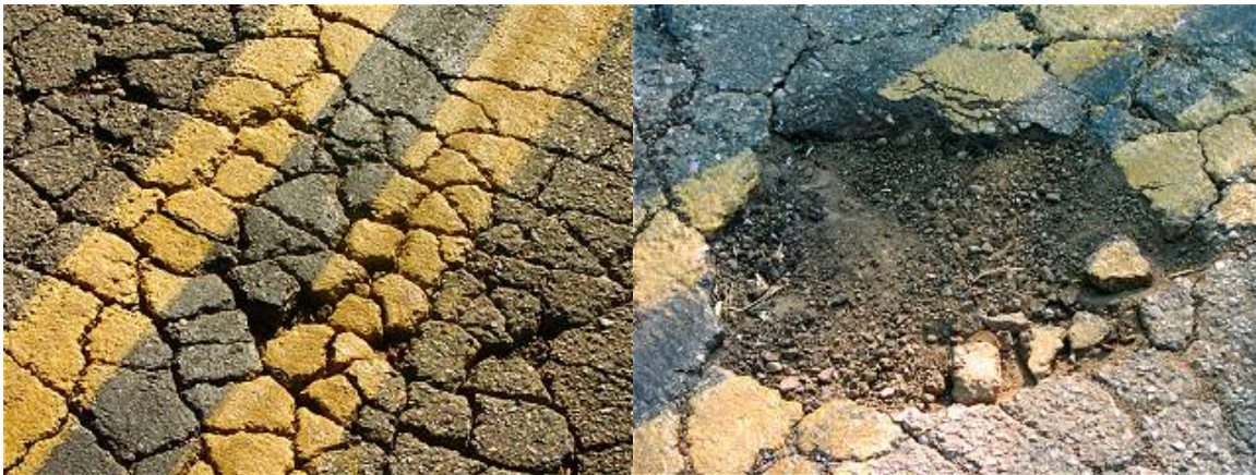
Figure 2. Alligator cracks and pothole formation
